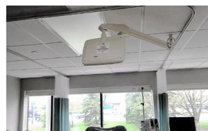
Suspended Ceilings or Glass Wall
